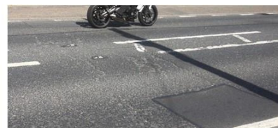
Non-intervention longitudinal cracking
